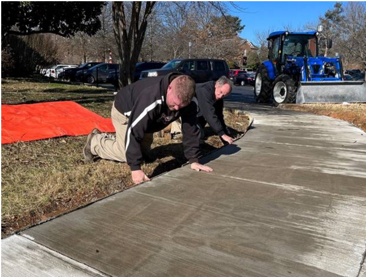
Chad Grindstaff, left, and Bill Fitzpatrick work on a newly constructed section of sidewalk.
